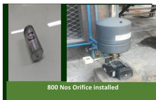
Figure 11. Booster pump installation.
